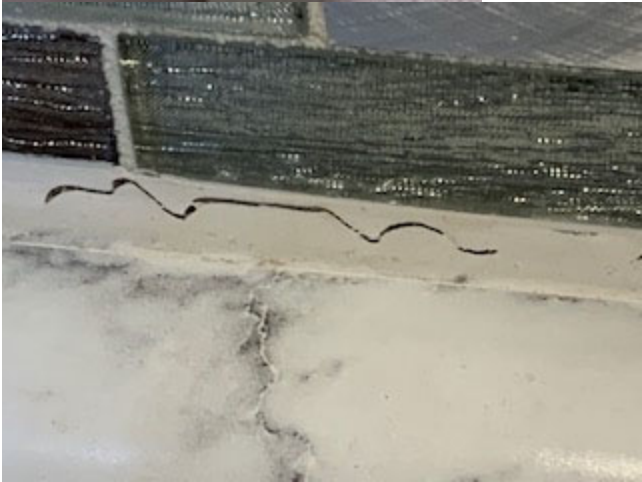
wromg grout used between backsplash and counter
